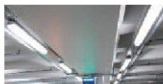
PLAFONIERE STAGNE IP65 LED CABLING
